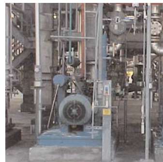
HP Stripper Bottom Equipment
