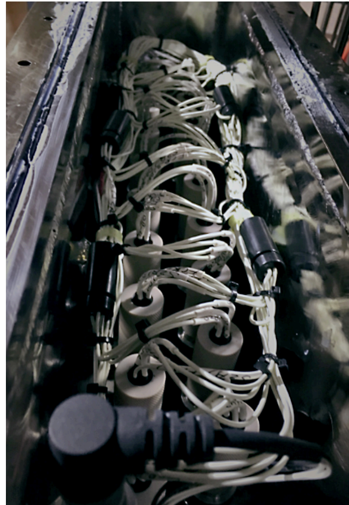
Greene Tweed's electrical harness installed in Baker Hughes' SeaPrime MUX Pod
